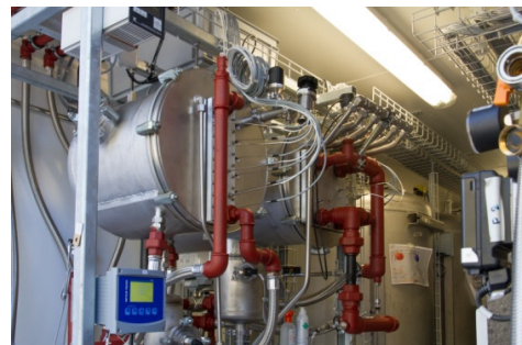
Fig. 4: Picture of the demonstrator heat and mass exchanger connected to the storage tanks.
