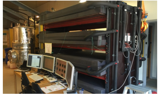
Fig. 16: PCM heat storage with four modules for the demonstration system.
